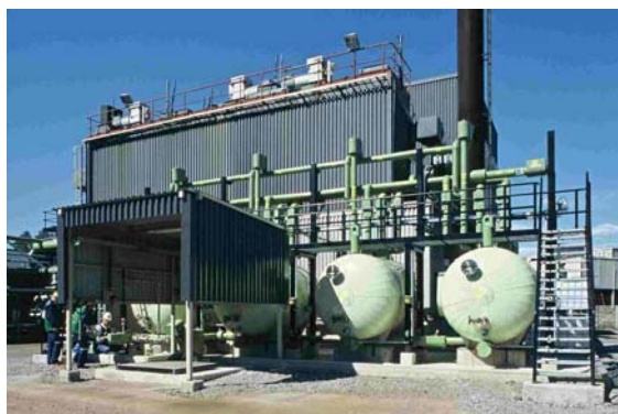
Figure 2. Product storage area of the pilot plant
